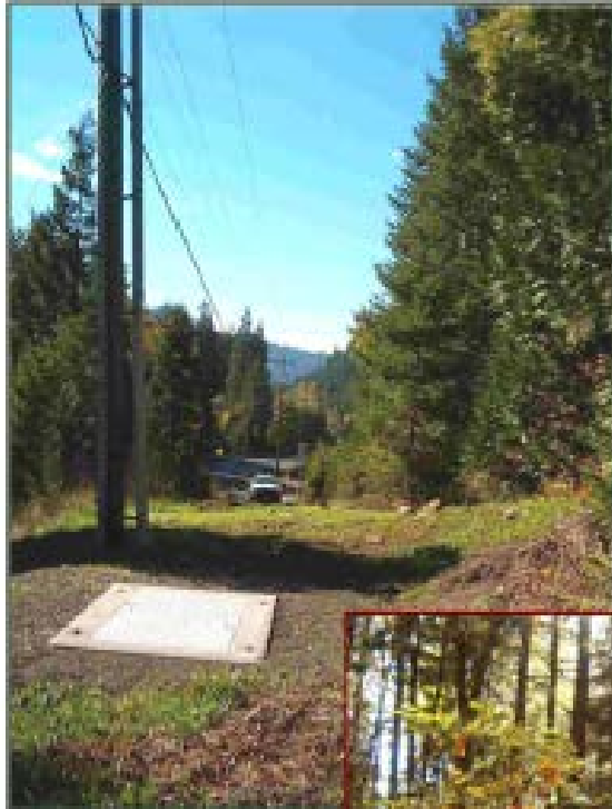
Top: Connection from overhead power to vault.
