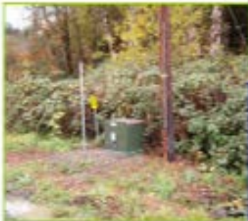
Top: Abandoned above ground line easement showing susceptibility to falling vegetation damages.
